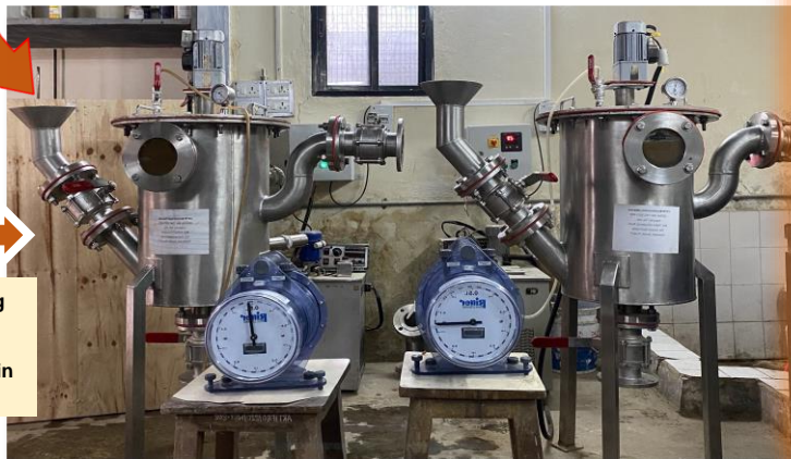
Biomethanation of rice straw in anaerobic digesters (60L)
